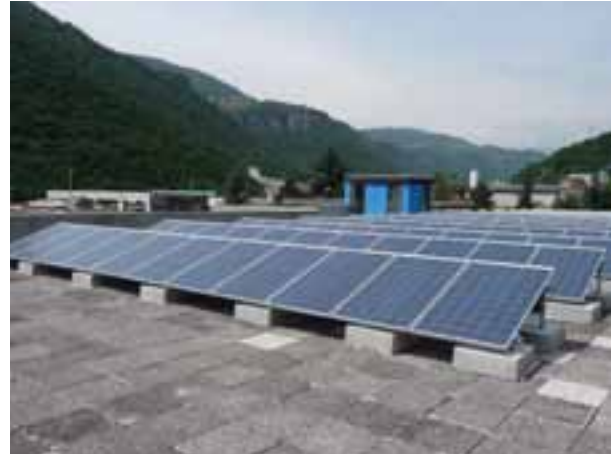
Figure 7 - Solar energy plant
