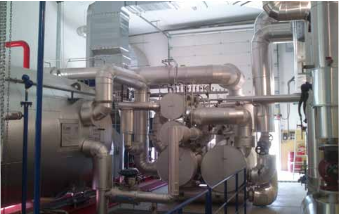
Figure 24 - Turboden 10 CHP SPLIT - ORC turbine
