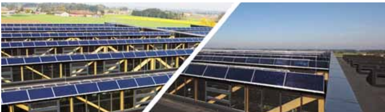
Figure 12 - Solar thermal collector area on the roof of the "SUN MASTER" production hall
