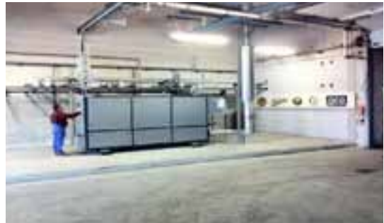
Figure 33 - CHP Plant/Power station. Supplier of the technology:Thermic Energy RZ GmbH
