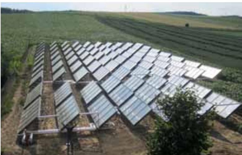
Figure 10 - Collector field of the solar process heat plant
