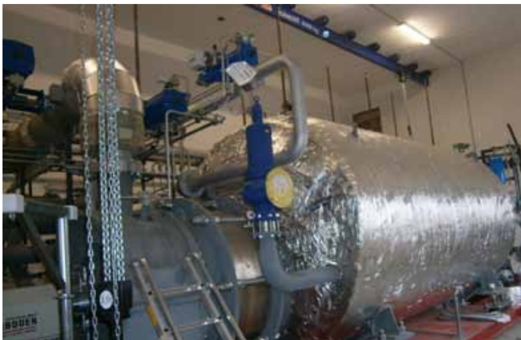
Figure 23 - Biomass thermal oil boiler
