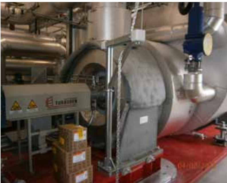
Figure 25: Turboden 10 CHP SPLIT - ORC turbine
