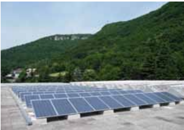
Figure 8 - Solar energy plant
