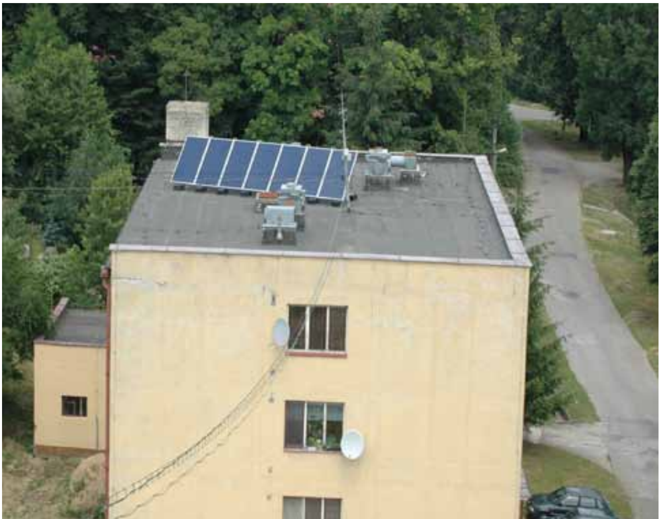
Figure 20: installed solar collectors
