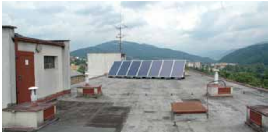
Figure 19 - Installed solar collectors
