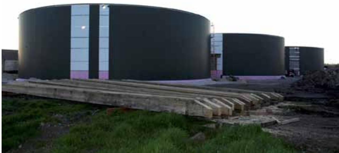
Figure 47 - Tanks for waste fermentation
